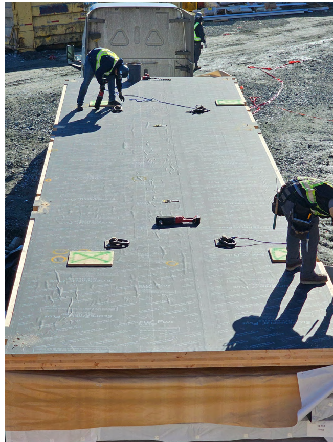
Figure 51 Panels are delivered to site and installed directly from the truck. The panels have a protection membrane installed to the face of the timber.
