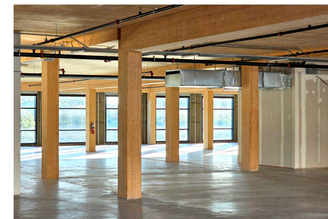
Figure 35 A fire suppression sprinkler system in a mass timber building. If the sprinkler system is used during occupancy, it will be necessary to identify locations where water may have traveled beneath the concrete topping.
