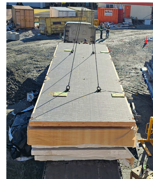
Figure 39 A CLT floor panel with a factory-installed membrane being hoisted into place at a project site.
