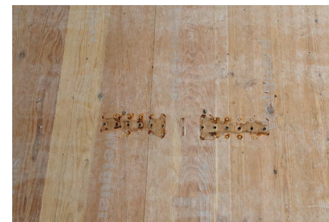
Figure 49 Holes in the protective membrane where a temporary fall protection anchor was installed. A membrane patch was not installed once the anchor was removed.
