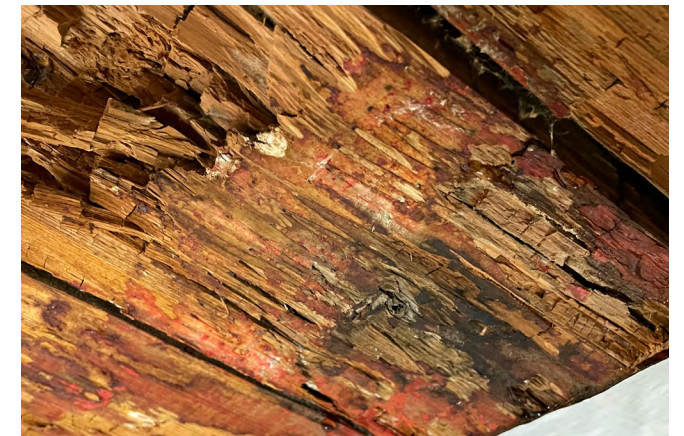
i) Severe deterioration of a CLT floor/soffit condition due to water intrusion from the wall above and the use of low-permeance membranes on both the top and bottom of the floor panel.
