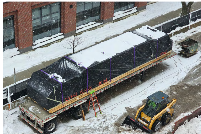
Figure 52 A mass timber panel is transported to the construction site on a truck bed. The mass timber is completely covered in a secure, heavy-duty tarp.
