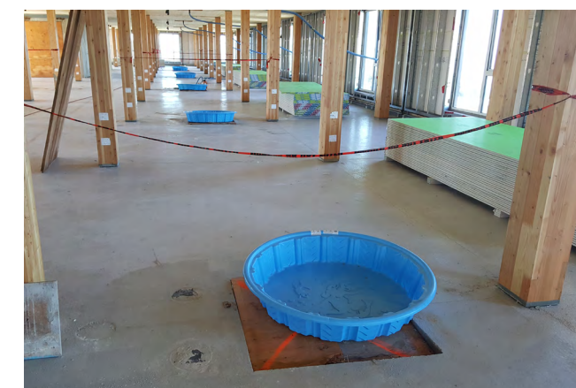
h) Water collection with kiddie pools (other collection devices like pails can also be used). The collected water is regularly removed from the building.
