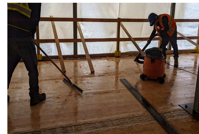
Figure 48 An on-site crew is mobilized to remove water from a mass timber floor using squeegees and shop vacuums.
