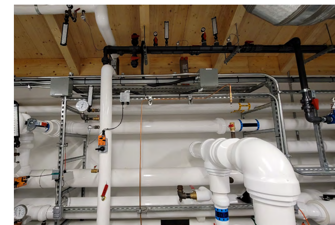
Figure 36 A mechanical room in a mass timber building. Installing targeted moisture protection at the mechanical room floor assembly, and regular inspection and maintenance of the equipment and piping, is recommended to reduce the risk of wetting the mass timber during occupancy.
