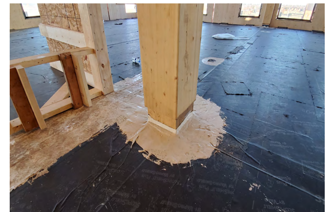
Figure 58 A temporary column detail that prevents water from traveling into the column connection.
