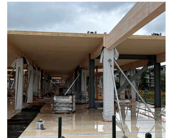
Figure 82 The protective membrane provided protection to the CLT and glulam even in very wet conditions.
