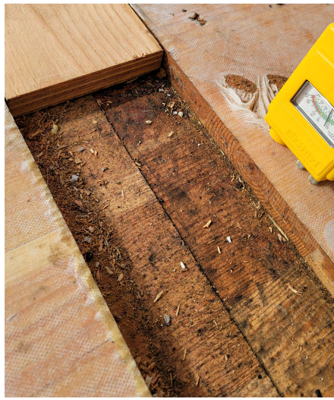
Figure 66 Mass timber joint with its spline removed and wet wood visible. Moisture was trapped undetected under the spline.
