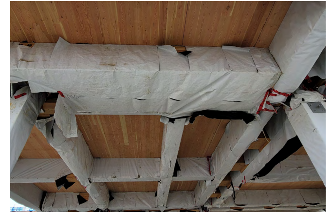
Figure 30 Glulam columns and beams protected using the factory wrapping. The factory wrapping is removed at structural connection, and the wrapping at the underside of beams and bottom of the column is opened to allow for water drainage.
