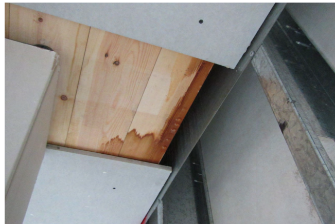
b) Moisture accumulation within a mass timber ceiling cavity due to the installation of interior gypsum board before the installation of adequate moisture protection on the floor panel above.
