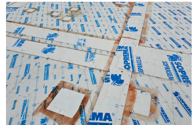
Figure 59 A mass timber roof where the protective membranes were regularly repaired and patched. Membrane patches and strips were installed over panel joints, areas of damage, and structural steel connections.
