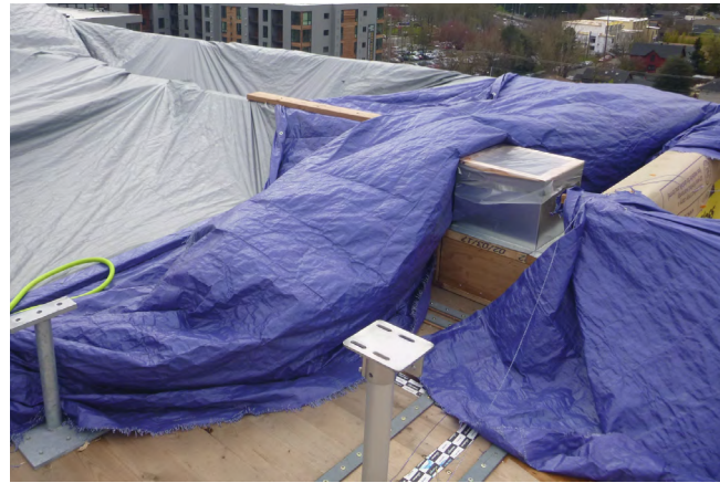
Figure 54 A tarp installed over the mass timber parapet at a roof has left a portion of the roof exposed and at risk of wind-driven rain migrating under the edges of the tarp. Water is not able to drain from the tarp, so removal with shop vacuums or pumps is required.
