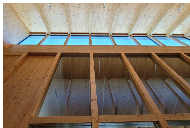
Figure 75 The underside of a mass timber roof and exterior windows that are a part of the building enclosure.
