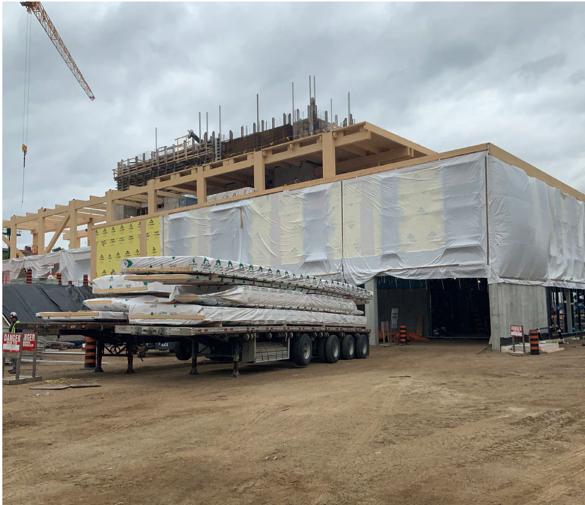
Figure 41 Mid-construction of the mass timber Science Collaboration Centre in Chalk River, Ontario. Perimeter hoarding is installed as each floor is completed to protect the mass timber from moisture exposure (Canadian Nuclear Laboratories).
