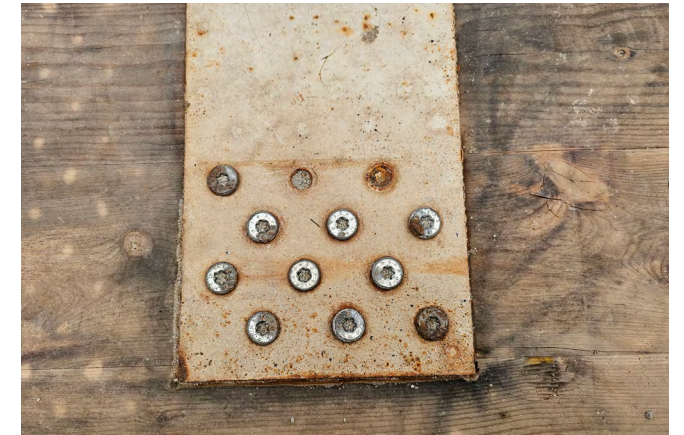
g) Failure of structural fasteners caused by swelling of the wood and corrosion on fasteners.
