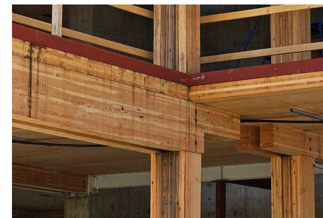
Figure 73 An example of staining caused by a reaction between iron and wood tannins in a mass timber project exposed to wetting from above.
