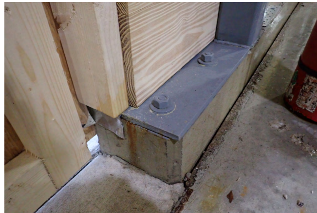
Figure 28 A CLT wall is installed onto a concrete curb to elevate the base of wall above grade level. The CLT and concrete curb are separated with a metal attachment.
