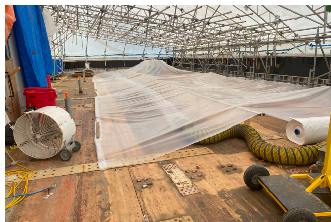
Figure 71 Localized drying under plastic sheets to address wet splines.
