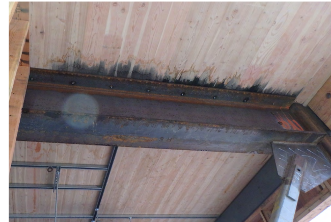
d) Visible staining on the underside of a CLT floor panel due to the damp wood being in direct contact with unfinished steel, resulting in a chemical reaction between the wood tannins and metal.
