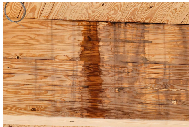
c) Staining on a CLT wall and intermediate floor panels due to ponding water on the floor panels above.
