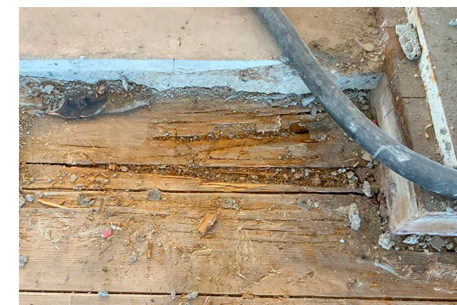
Figure 7 A CLT floor with concrete topping removed to reveal decay of the wood.
