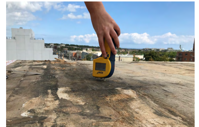
h) Microbial growth and deterioration of an unprotected CLT roof panel.
