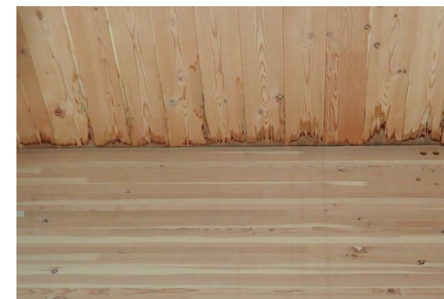
Figure 72 An example of general wood staining caused by wood tannins migrating with the water in a mass timber project exposed to wetting from above.
