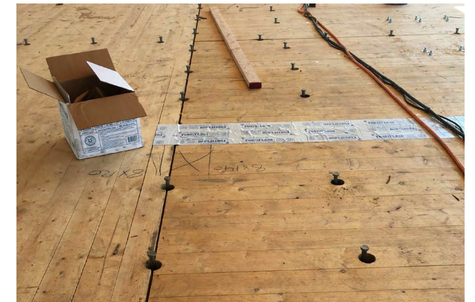
Figure 22 Timber-concrete composite CLT floor with shear connectors installed prior to concrete pour.
