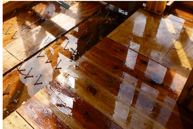
a) Moisture ponding on and absorbing into a timber-concrete composite (TCC) floor panel before the concrete is scheduled.
