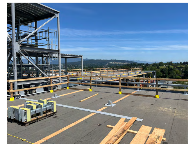
Figure 45 Factory-applied roofing base sheet moisture protection over CLT at the roof level.
