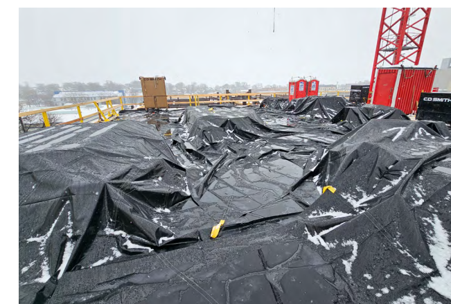
i) A tarp used to collect snow, which is then removed from the building using the overhead crane.
