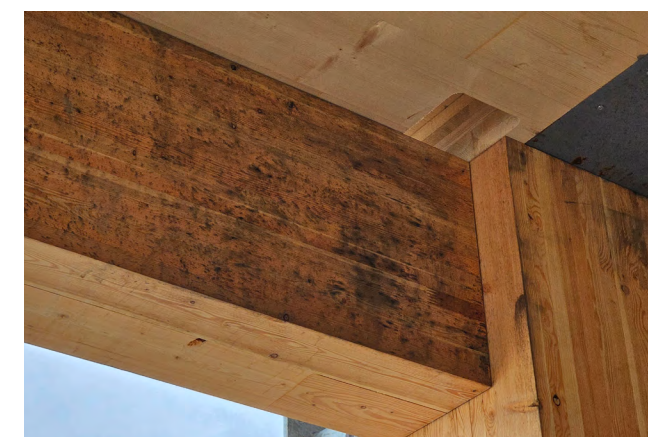
Figure 50 Mass timber beam with discolorations caused by staining from iron filings.
