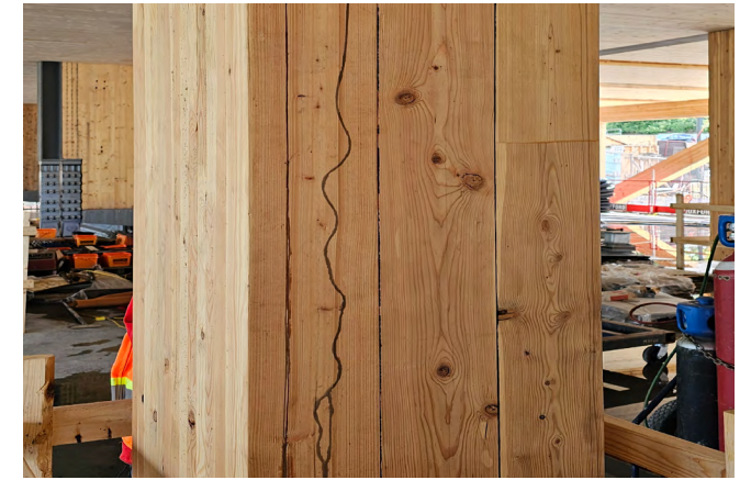
Figure 29 A glulam column with dark iron staining from water traveling down the column from the level above.
