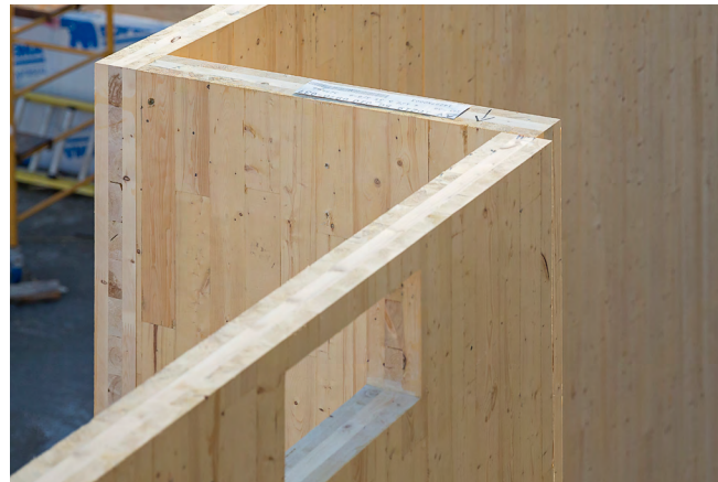
Figure 27 CLT wall panels with exposed penetrations and rough openings prior to on-site application of a WRB membrane.
