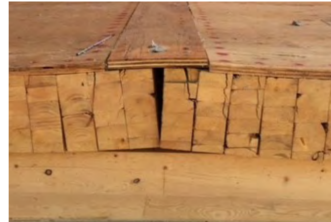
f) Built-up timber panel damage and distortion resulting from moisture-related panel expansion.
