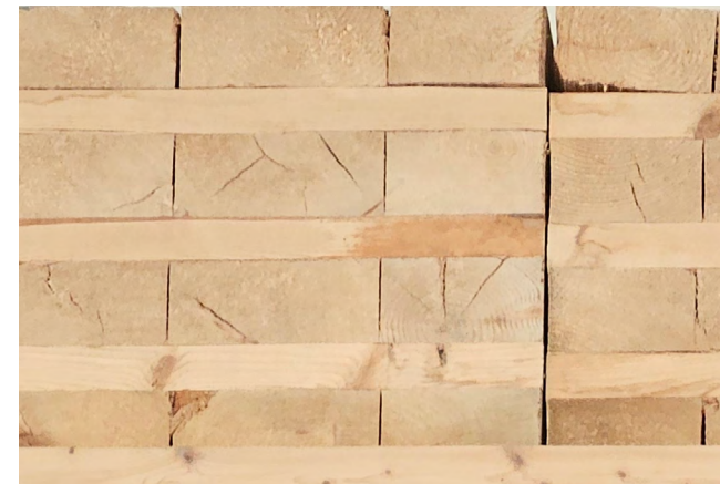
e) Checking of CLT due to repeated wet-dry cycles.
