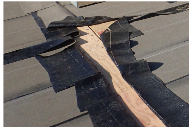
Figure 13 A mass timber roof assembly. Once all laps of the membrane are sealed, the air and vapor barrier membrane visible in this photo will temporarily protect the mass timber from moisture (Catalyst, Spokane, WA).
