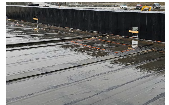
Figure 16 A sloped CLT roof panel with a vapor-impermeable roofing base sheet acting as the moisture protection membrane during construction. The membrane will act as the base ply of the final 2-ply roof membrane. The panel slopes to the roof perimeter.
