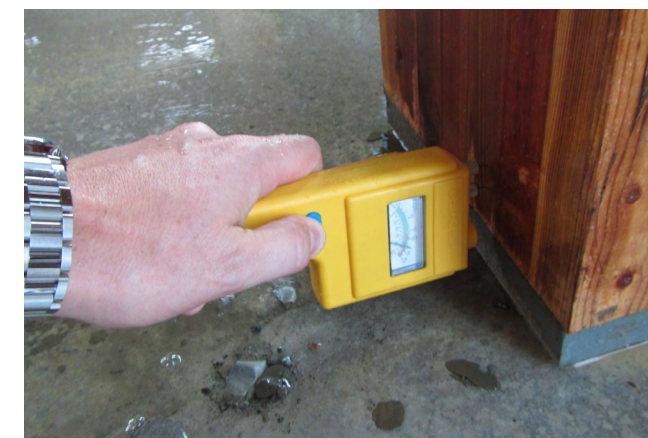
Figure 64 Moisture content reading taken at the base of a mass timber column that has been exposed to moisture.
