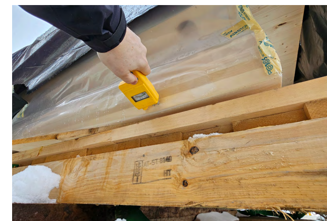
Figure 65 A worker takes a moisture content reading of a CLT panel that is stored on-site as part of the regular monitoring requirements outlined in the project's moisture management written plan.
