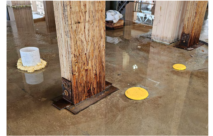
Figure 31 Water absorption at the base of a parallel strand lumber (PSL) column due to contact with wet surface conditions.
