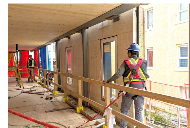
Figure 8 A mass timber building with prefabricated wall panels being installed prior to concrete topping placement.
