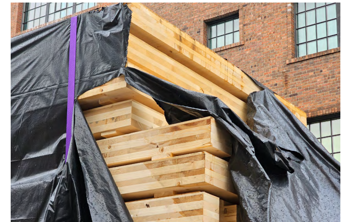
Figure 53 CLT panels covered in plastic when stored on-site. The plastic was not durable and not secured, leading to the exposure and wetting of the stored panels.
