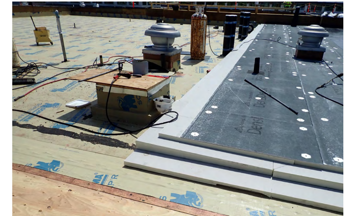
Figure 17 A roof assembly with mechanically fastened insulation and coverboard system. The fasteners are installed through the membrane, which acts as the construction phase moisture protection and the permanent air and vapor barrier.
