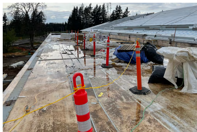
Figure 61 Mass timber roof where ponding water is not being removed. Water has gotten underneath the protective membrane through laps and areas of damage to the membrane, resulting in wet mass timber and staining.
