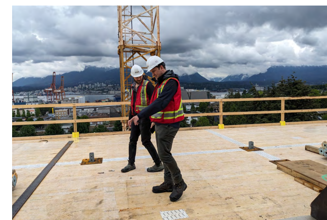
Figure 63 Visual inspection of mass timber floor during the construction phase to identify areas of damaged membrane, trapped water, etc.
