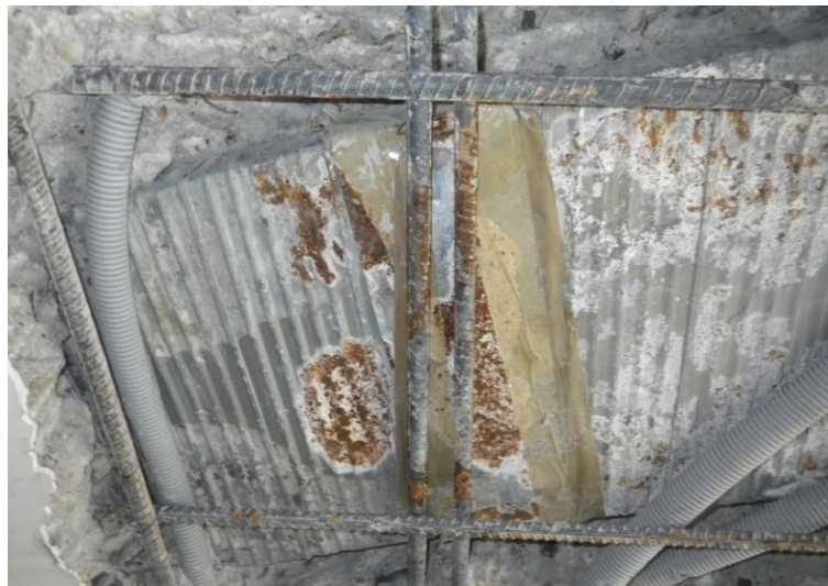
Figure 3.4: Photo of a chip and replace repair. Work consisted of mapping out the concrete reinforcing, chipping away the concrete in the suite above and below the duct, sealing the duct with liquid-applied sealant, replacing the concrete, and repairing the interior finishes.
