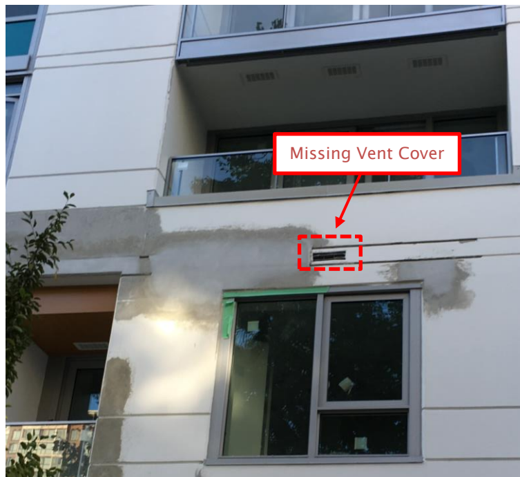
Figure 3.1: Photo of the exterior of a building with the exhaust vent cover removed (red), exposing the duct to rain.
