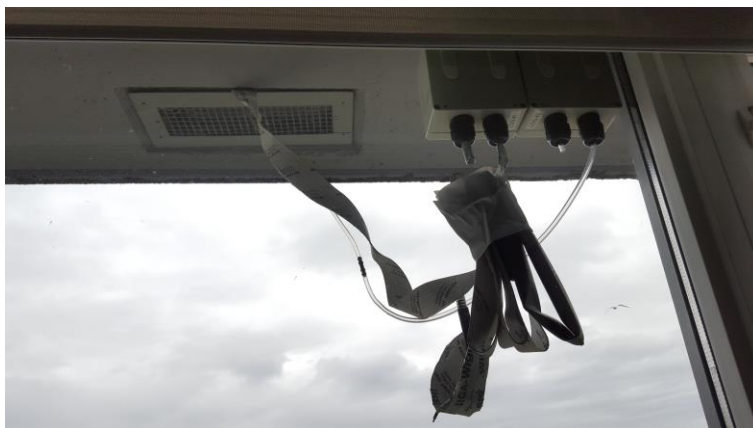
Figure A.2: Photo of the sensor intallation at Site A. Dryer exhaust vents under a soffit.
