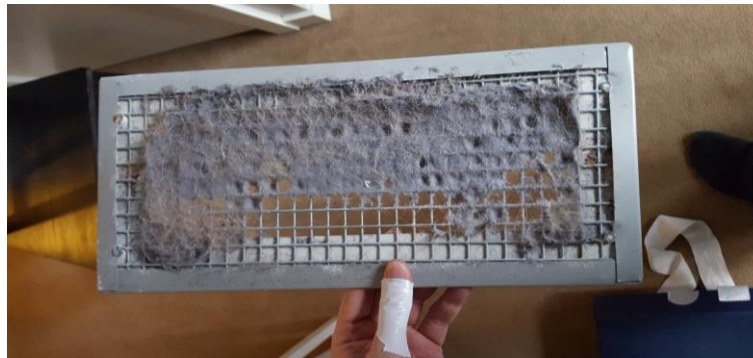
Figure 3.3: Photo of an exhaust vent cover with extensive lint buildup. Grilles and exhaust ducts should be cleaned regularly.
