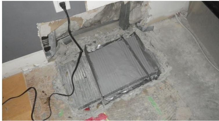
Figure 3.2: Photo of a duct which has been remediated by chipping out the concrete and sealing the duct with liquid-applied waterproofing. Extensive work to both the suite above and below was required in order to carry out the repair.
