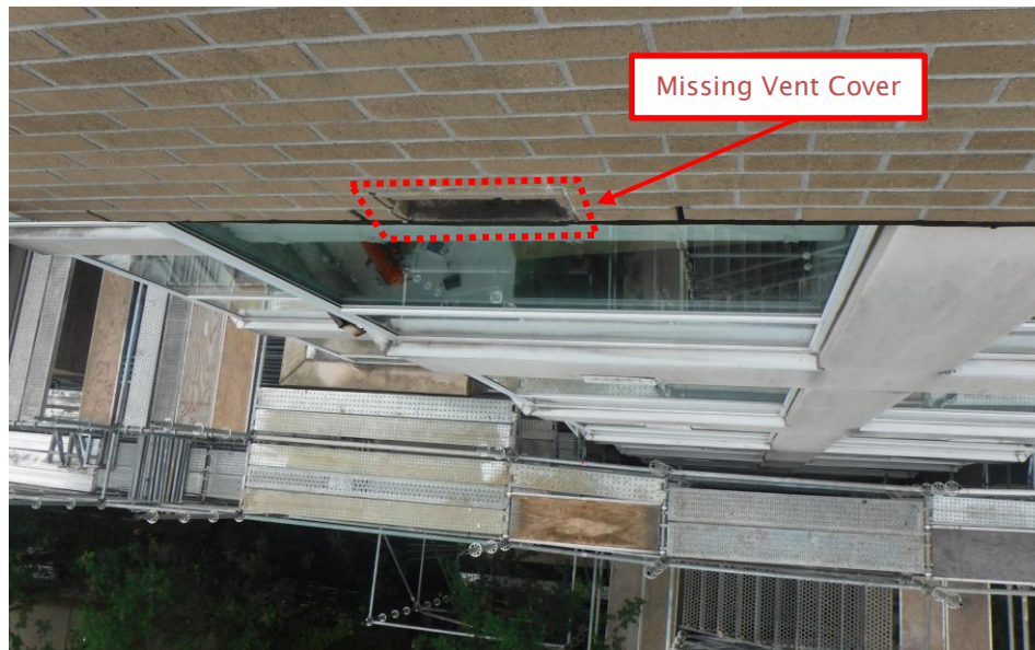
Figure 1.10: Photograph taken of a wall from above showing an exhaust vent opening. Note the vent cover has been removed and the duct is therefore exposed to rainwater.
