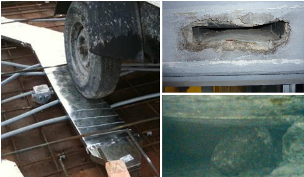
Figure 1.2: In-slab duct damaged during construction (left & upper right), and damaged during concrete pour (bottom right)
