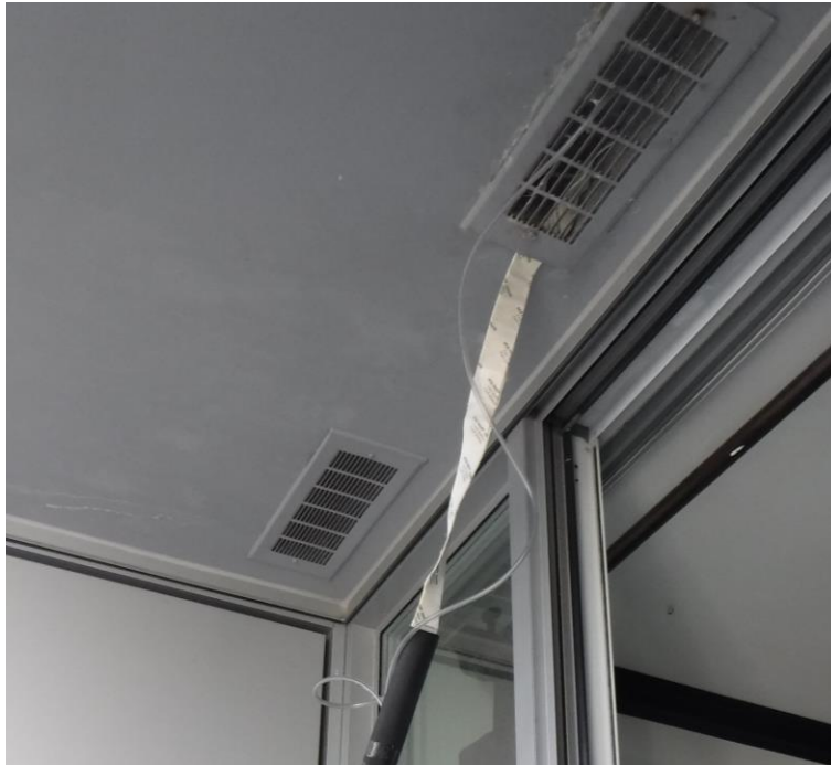
Figure A.11: Photo of the sensor installation at Site C. Dryer exhaust vents under the exposed concrete balcony of the unit above.
