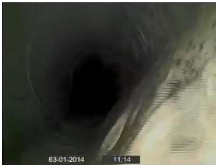
Figure 1.8: Screen capture taken from a borescope video of an in-slab duct with severe moisture buildup. Note the standing water (> 1" depth) on the bottom right corner of the image (bottom of the duct).
